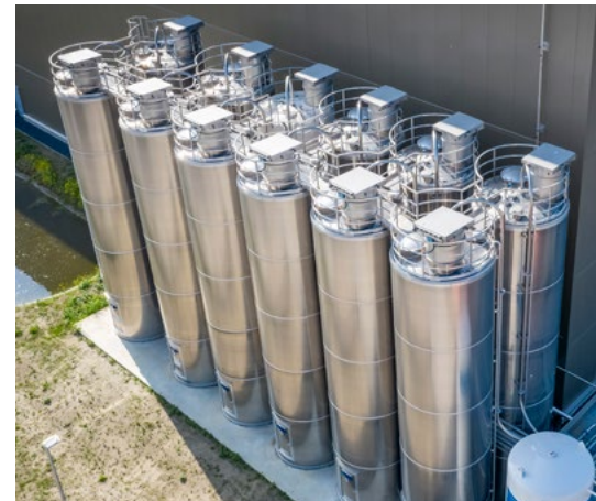
Visible from afar: the 12 outdoor silos for storage of the main components.
