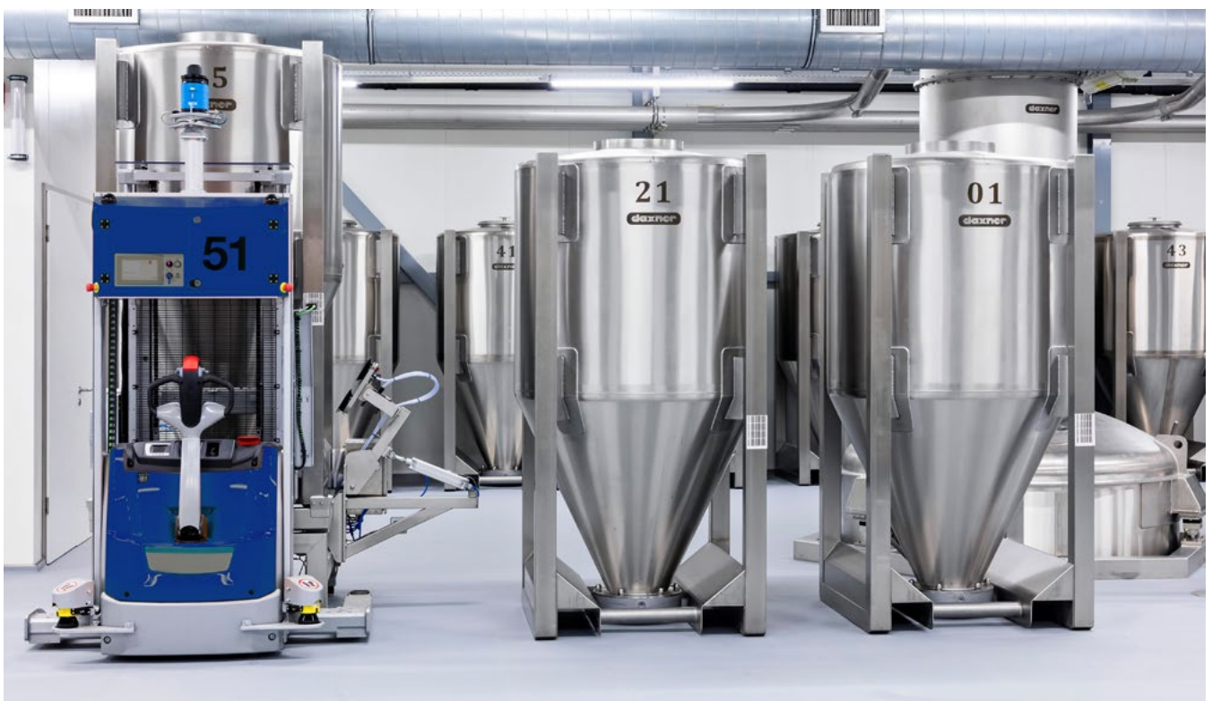
The containers move through the plant with the help of Automatic Guided Vehicles.
