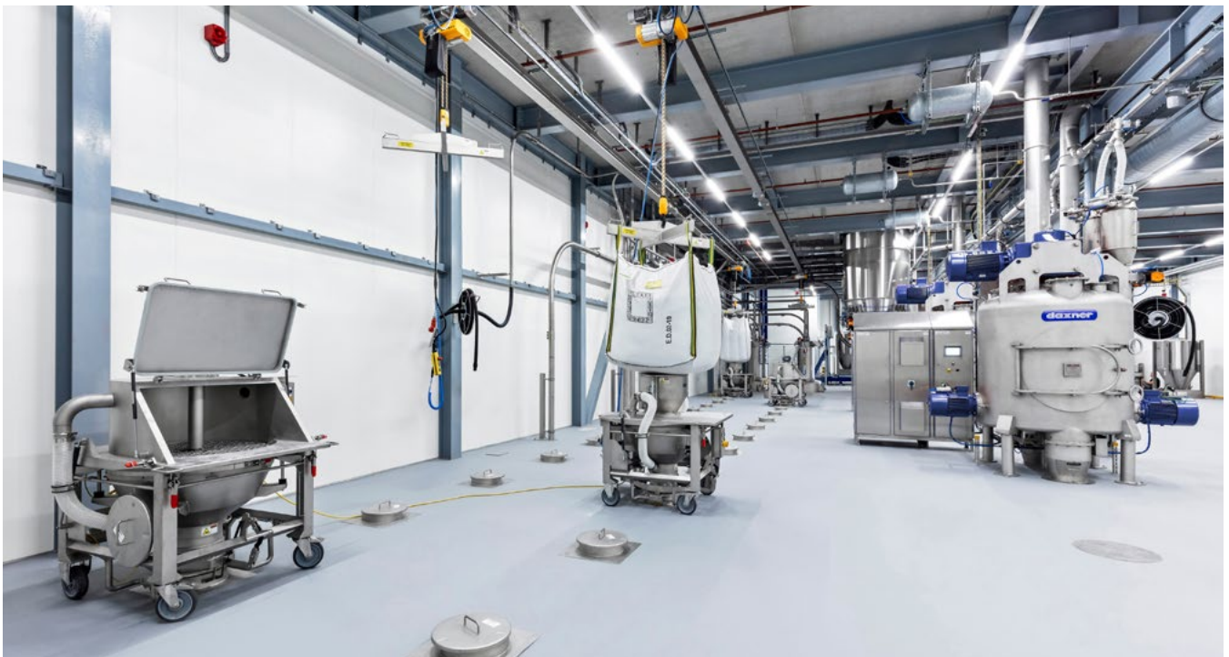
Contamination free filling of the day bins with big bags. On the right: vertical mixer in hygienic design.
